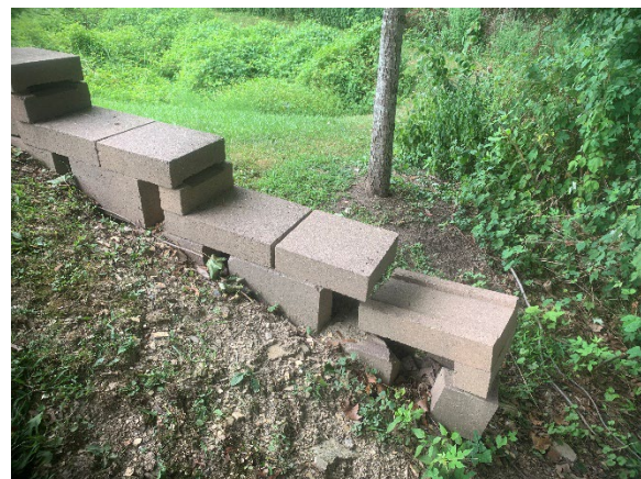
The retaining wall appears to need maintenance as the result of a collision or shifting ground.
