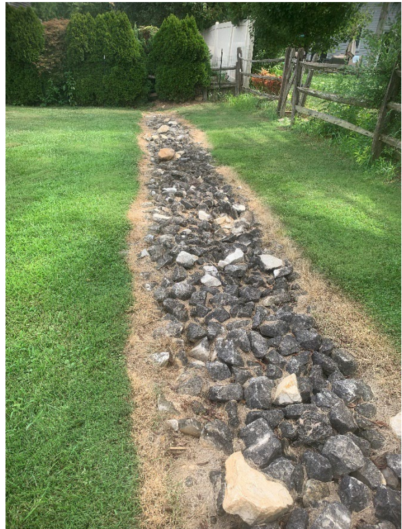
Erosion channels have formed in the lawn. Treated with stone, they will continue to erode unless the stormwater itself is managed.
