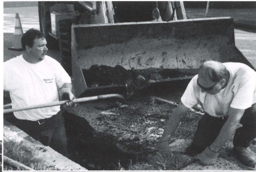
Top: Stormwater drain upkeep is one of the Public Works Department's critical tasks. Crews regularly clear the tops of drains, paying particular attention to clearing debris prior to severe storms. Capital projects, such as the repair on Revere Road are regularly scheduled to keep the infrastructure functioning. From left: Chuck Gehringer, George Kobi
