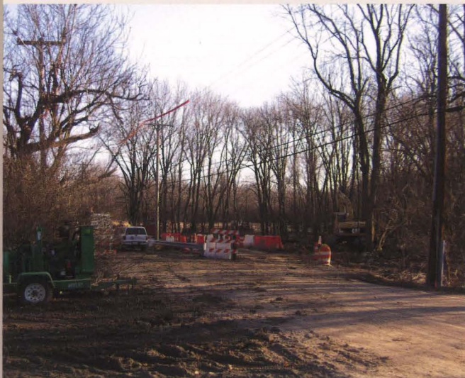
The new drainage culvert being installed at Lorraine Run on West Valley Green Road in Fort Washington.
